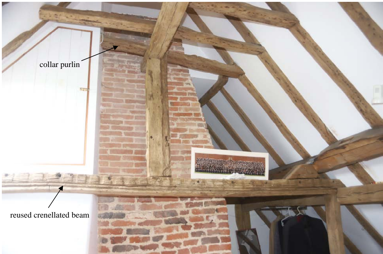
Additional queenpost truss inserted in 17th century to support truncated collar purlin with a re-used crenellated beam for the collar
