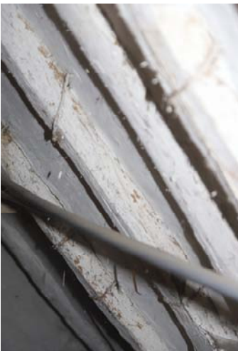
Fig 7: Narrow pole rafters suitable only for thatch
