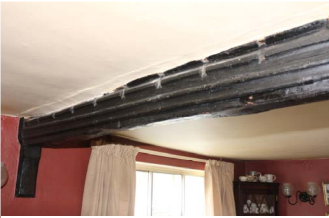
Fig 3: North side of moulded beam BB' on ground floor with crenellated moulding. The stud partition below the beam has been removed
